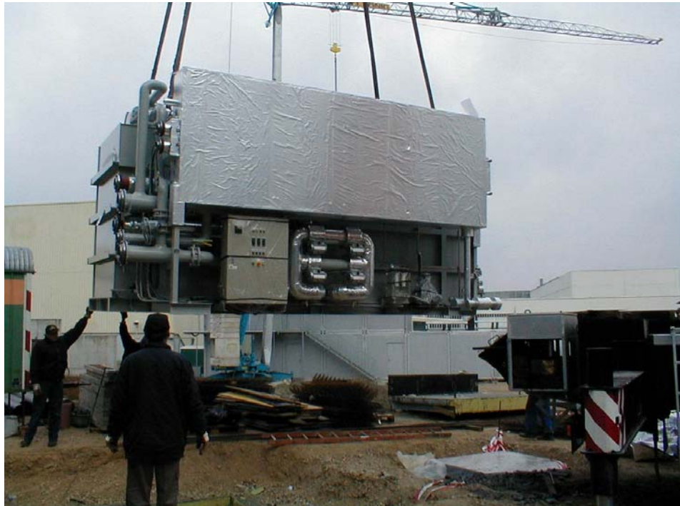
Figure 5. Photo of a 0.5 MW Mycom adsorption cooling machine, of double size of the demonstration plant planned for Helsingborg /Mycom; Albring/.
