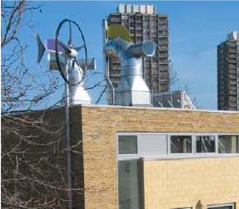
An urban wind turbine in the UK
