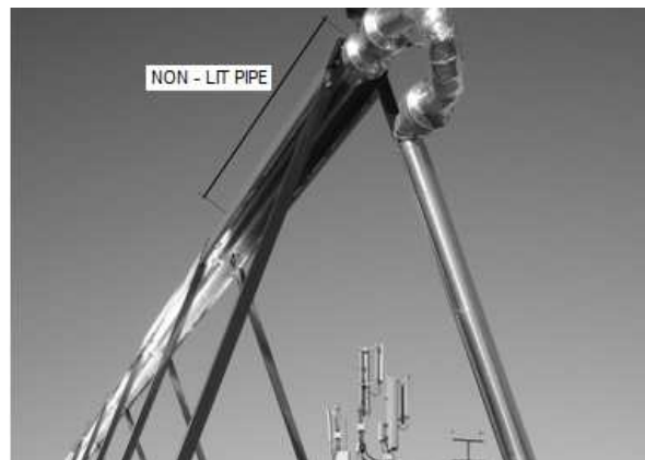
Figure 4. Non – lit pipe due to azimuth.
