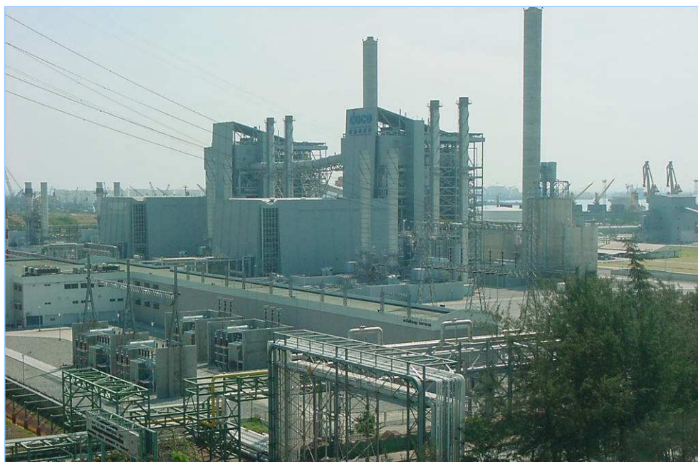
Figure 5: Third phase of the CDE installation in Map Ta Phut industrial estate
