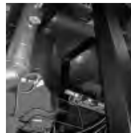
12 Ostfildern, Stuttgart. The biomass plant: detailed internal view of the machines
